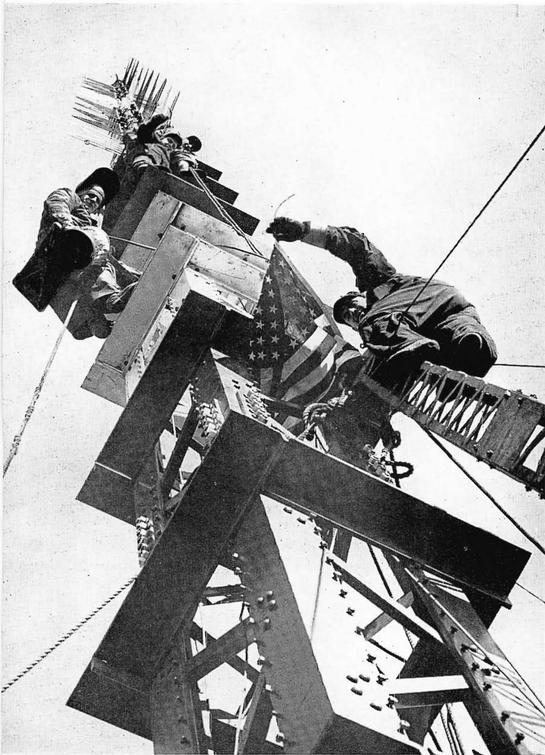
FIG. 4. Photo showing a closeup of the "multiple-use" TV antenna supporting tower located atop the Foshay Building. The seven diaphragms on lower portion are for strengthening and permit supergain elements to be mounted in between them.
