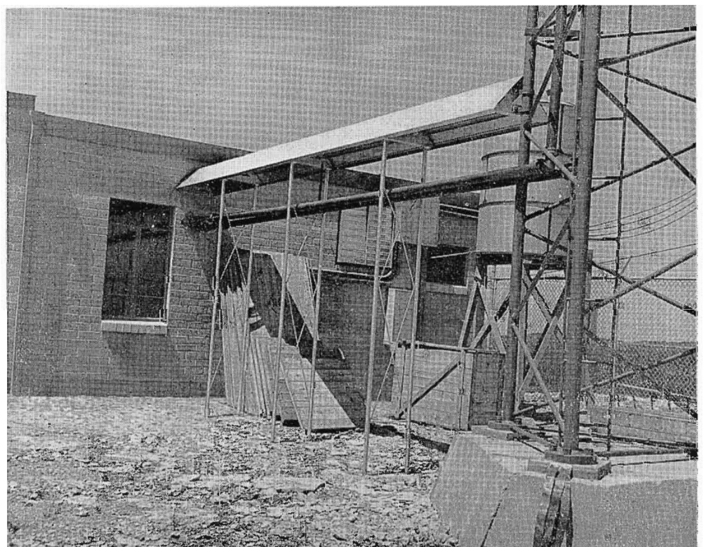
FIG. 9. View showing ice-deflecting canopy over transmission line run to tower. The line from building exterior to a point near the antenna is 3\frac{1}{2} " 50 ohm ultra-low-loss UHF Teflon line. MI-19089-9 50 ohm to 51.5 ohm transformers are used at antenna and building ends for impedance matching. Note transformers at the building wall.
